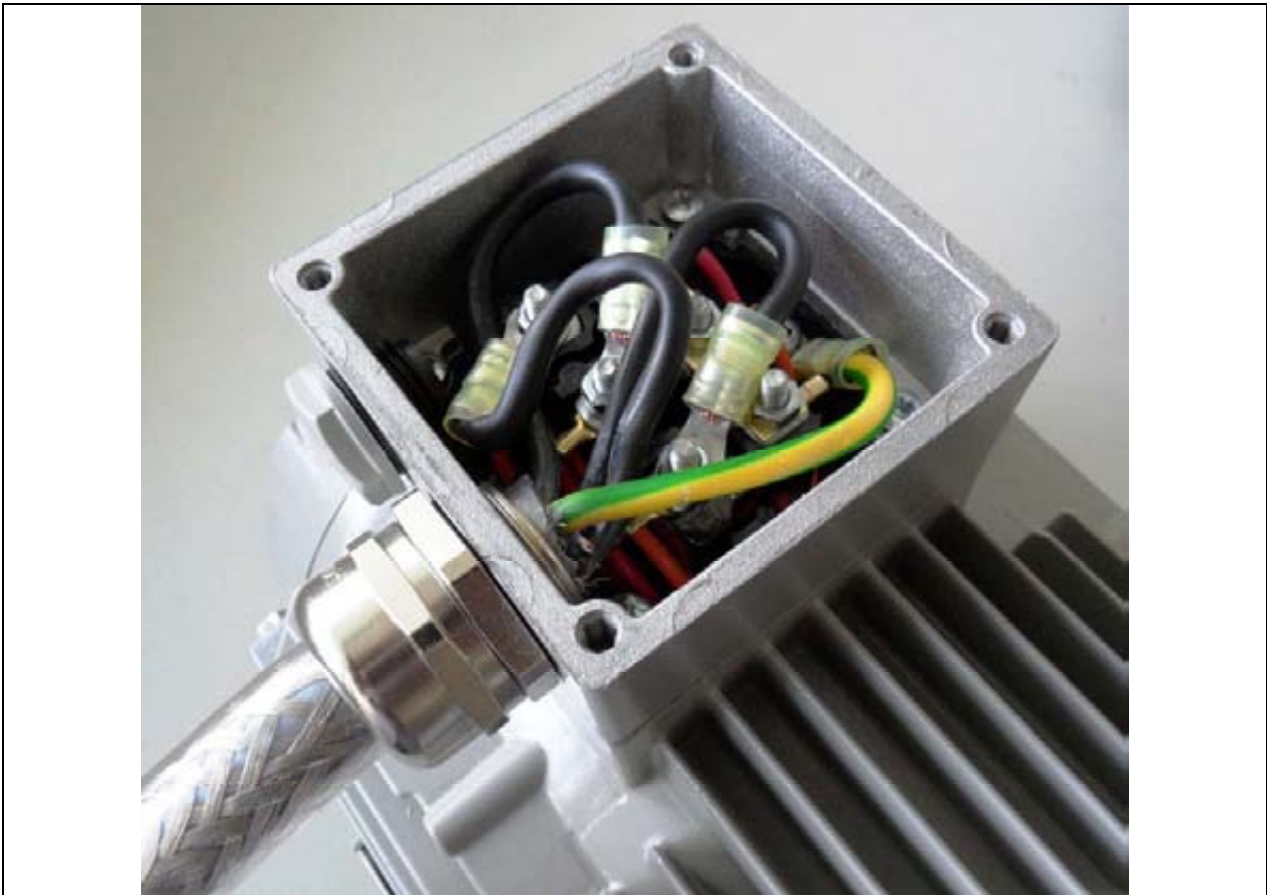
Fig. 7: Wiring on the motor connection box
